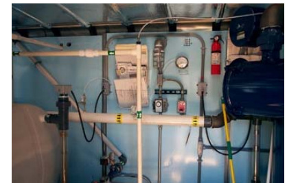
Photograph of AES' groundwater treatment system.
