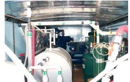
Photograph of groundwater treatment system.
