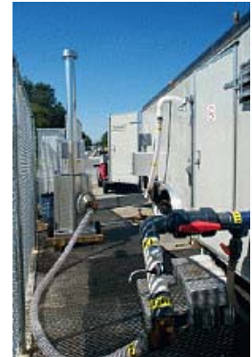
Photograph of the groundwater pump and treatment and SVE remediation system onsite
